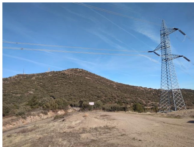
Fig. 6 Infrared and visual image of the 400kV overhead line proposed as the gateway location in the Sierra de Algairén.
